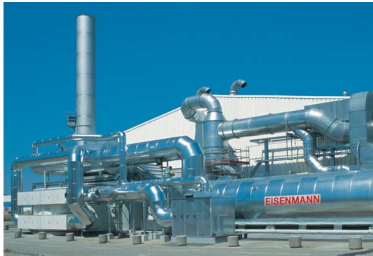
Adsorption wheel with thermal oxidation system for the treatment of exhaust air from a chemical production site
