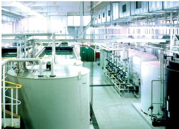
Complete waste water treatment for a car plant
