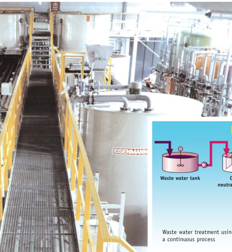
Figure, left: Chemical storage, continuous neutralization with a clarifier, batch reactor and DI water circulation system for an aluminium processor
