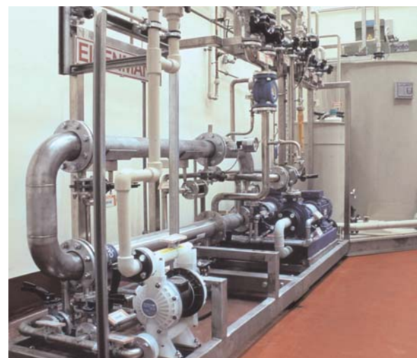
Ultrafiltration with tubular modules for printing ink recycling
