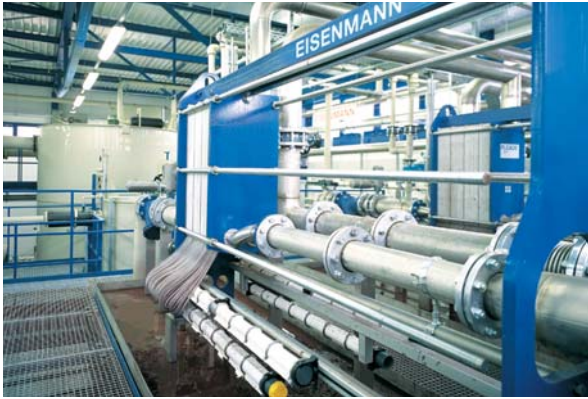
Cross-flow membrane filtration in the bypass to the bioreactor for biomass concentration and separation
