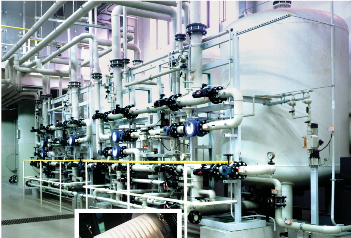
Sand filter installation for suspended solids removal
