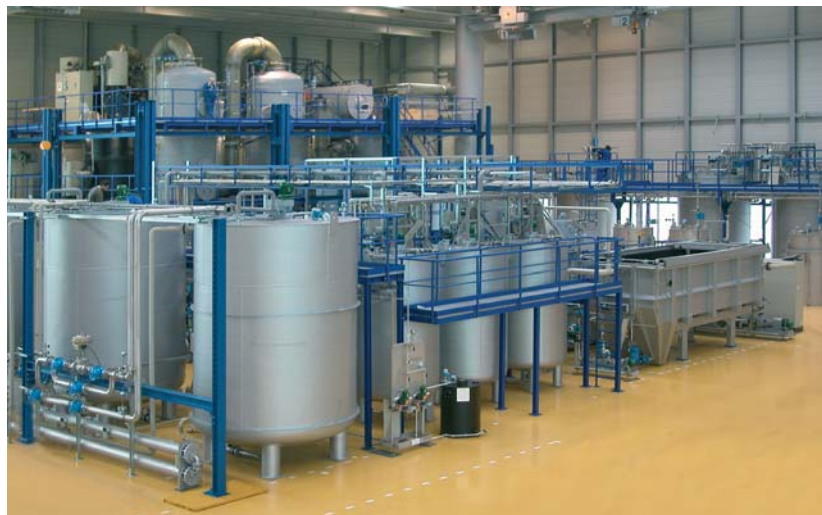
Disposal system for toxic wastes: In the background the thermal treatment and the exhaust air purification, in front of the waste water treatment plant. The total system was completely pre-assembled and commissioned at EISENMANN.
