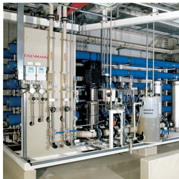
Reverse osmosis plant for water desalination
