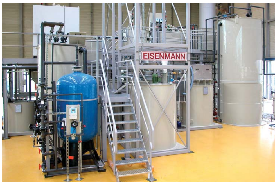
Continuous waste water treatment plant for fluorid removal, preinstalled and commissioned at EISENMANN
