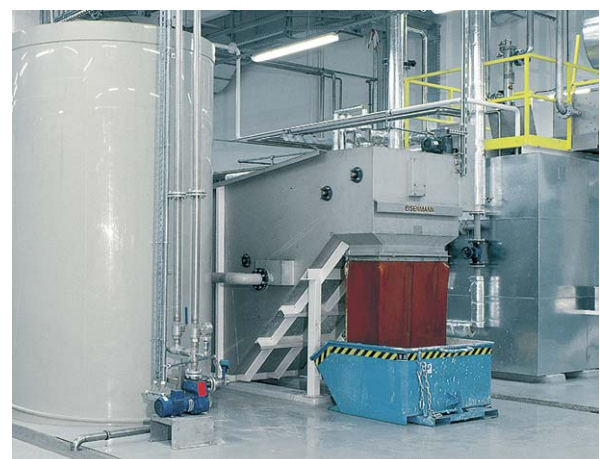
Paint sludge flotation in an EISENMANN flotator in an automotive plant
